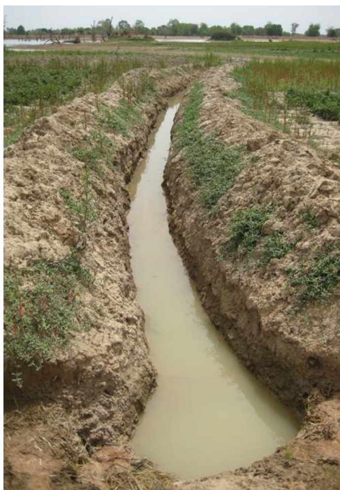
Creating a river diversion need not be sophisticated. Here, a simple channel for diverting river water has been dug in the mud.
