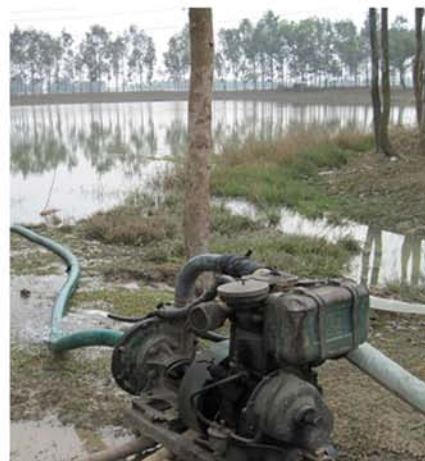
A motor pump is just one of the options to help farmers improve irrigation.
