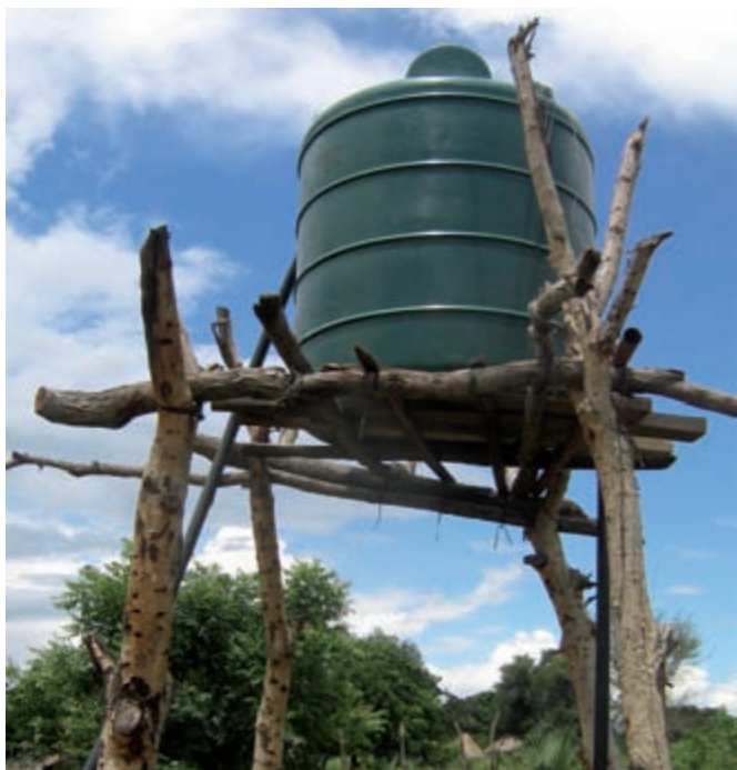
Figure 5: AWM as a storage tank which automates pressure for irrigation
