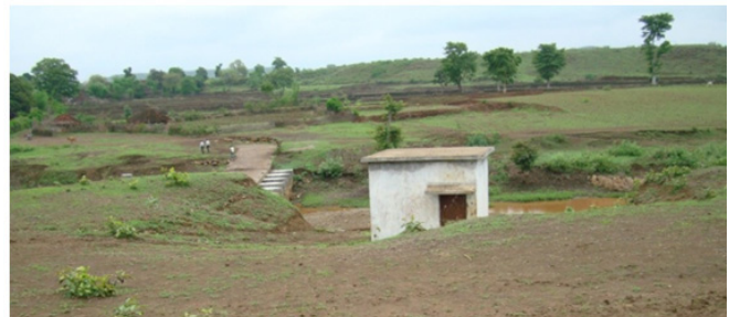
A pump house but no pump to install
