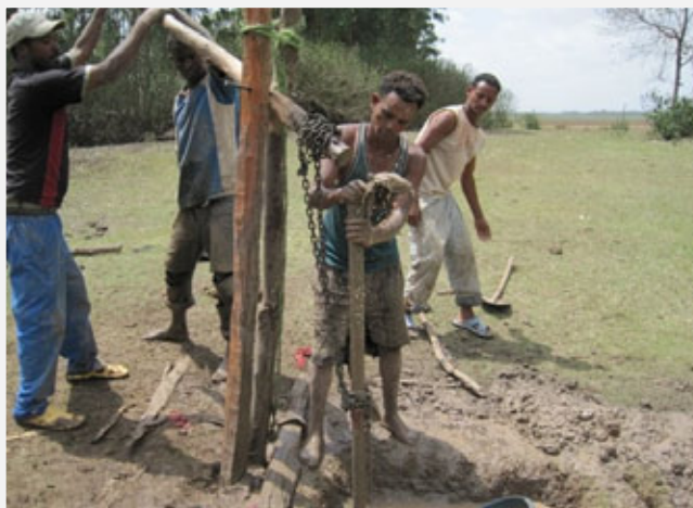
Well drilling is done by teams using manual labor and simple technologies.
