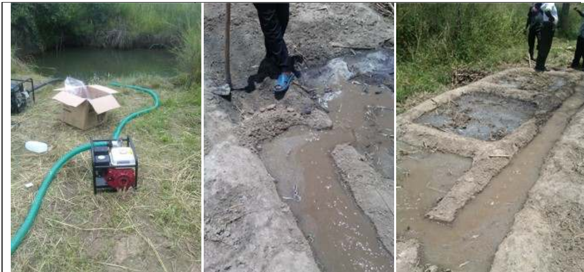
Photo 3: Testing a small motor pump to draw water from a nearby well. Photo: AWS.
